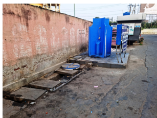
Figure D: unhygienic surroundings of Public Toilet
