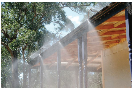
Figure 2: Exterior sprinkler system. This sprinkler system has the added benefit of protecting the outside of the building as well as the inside (Blaze Control). 13
