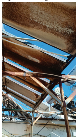
Figure 17: Rust on the steel structure of a solar panel. The image shows the negative impact of using a steel structure in an environment with high humidity.
