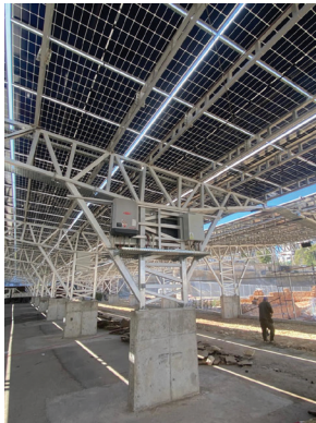
Figure 29: Anchoring is used in a solar park. The image shows the use of aluminum for the structure and anchoring of solar panels.
