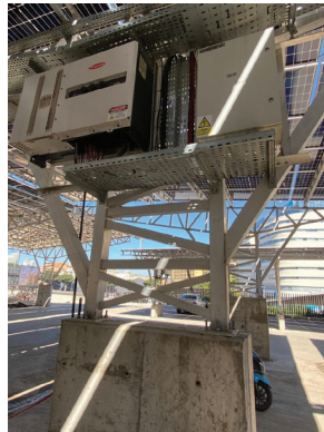
Figure 30: Battery installation in a solar park. The image shows an installation of a battery with covered wiring.
