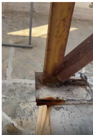
Figure 18: Rust on the anchoring connection of a solar panel installation. The image shows the impact of rust on the integrity of the anchoring system.
