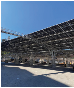
Figure 27: Solar Park installation. The image shows an example of an installed solar park.
