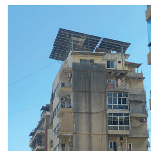
Figure 20: Solar panel installation on the edge of the rooftop. The image shows the installation of solar panels extending beyond the rooftop, which poses safety issues.
