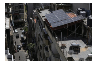
Figure 22: Exposed wiring of a solar panel installation. Image shows the lack of safety measures as wiring used is exposed to weather elements.
