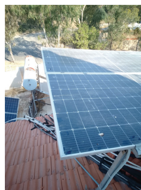
Figure 23: Covered wiring of a solar panel installation. The image shows the use of covered wiring in the installation of solar panels.
