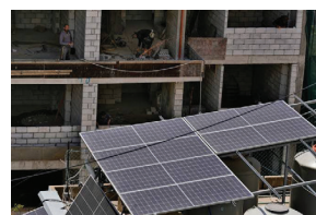
Figure 25: Solar panel installation over water tanks. The image shows the lack of planning in space use on rooftops and the installation of solar panels and wiring over preexisting water tanks.
