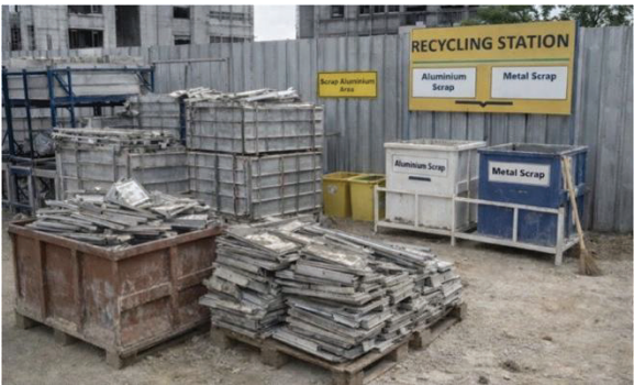
Figure 12: Scrap aluminum storage and recycling arrangement on site supporting circular economy practices.
